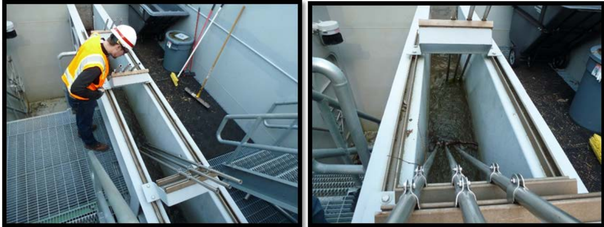
Figure 6-13. Inclined Debris Bars (North Fork Fish Collector)
