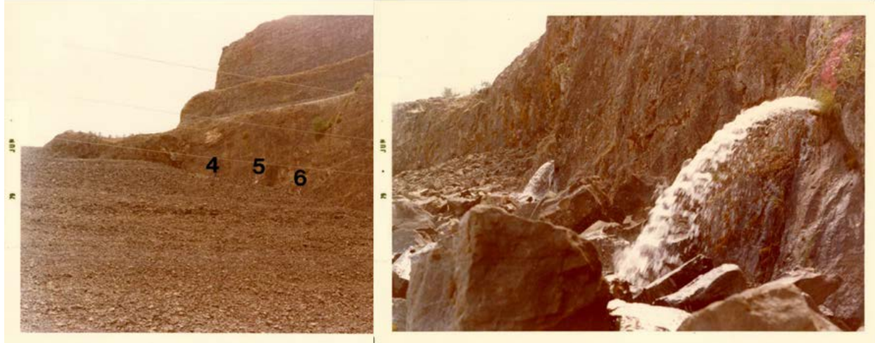
Figure 10-6. Left Abutment Horizontal Drains Locations (top) and Observed Flows in Drains 4, 5, and 6 (bottom)
