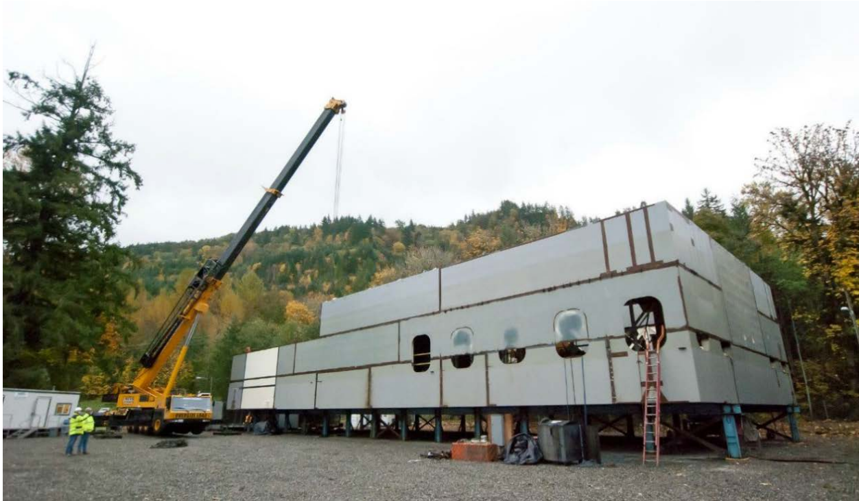
Figure 14-3. Lower Baker Floating Surface Collect Being Assembled at the Shore of Lake Shannon by Skanska
